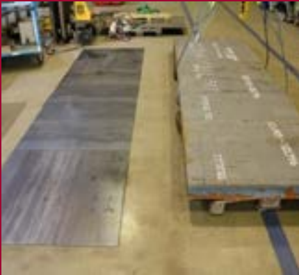
1. Place heat protection for the floor (if you have a heat sensitive floor)
